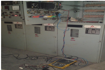
AIRCOSAVER equipment being tested at IIM Lucknow, Noida Campus
